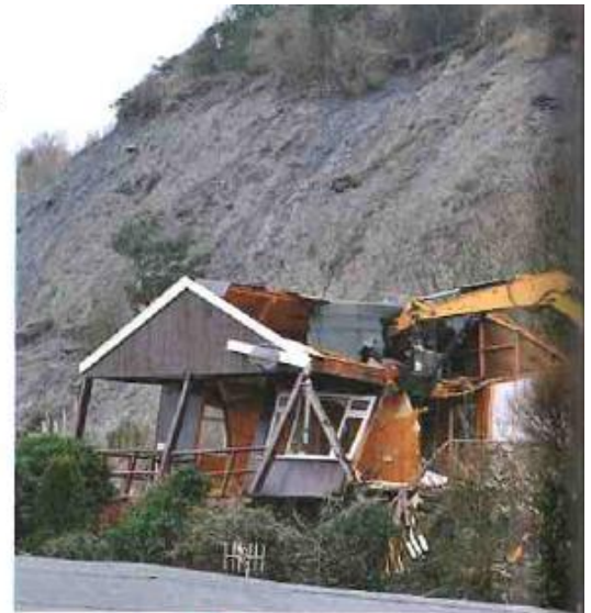
▲ Figure 1 One of seven holiday chalets that had to be demolished and removed from this location at Lyme Regis in 2014, following a series of landslips
